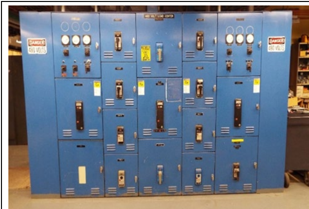
Photo 1: Electrical switchgear in Building 606 North
