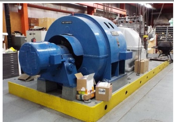
Photo 2: Electrical generator (foreground, blue) and turbine (behind generator at right) associated with the original operation of SM-1A in Building 606 North
